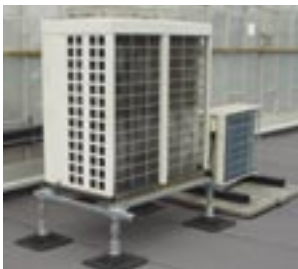
Plant & Equipment Support System
